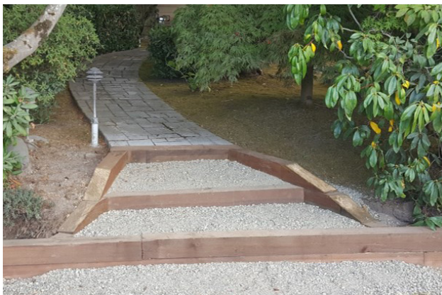
Example of Landscape Restoration on 91 st Avenue – Timber Edging Throughout the Site Was Added to the Project via a Change Order
